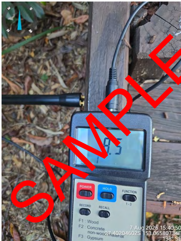
P01 - Moisture reading of 8.5% to accessible external timber.
