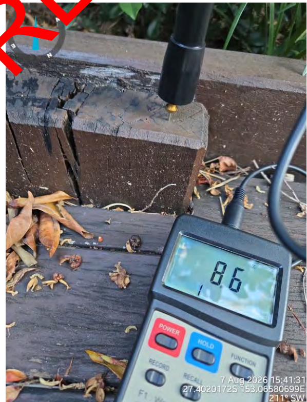
P02 - Moisture reading of 8.6% adjacent to visibly cracked timber.
