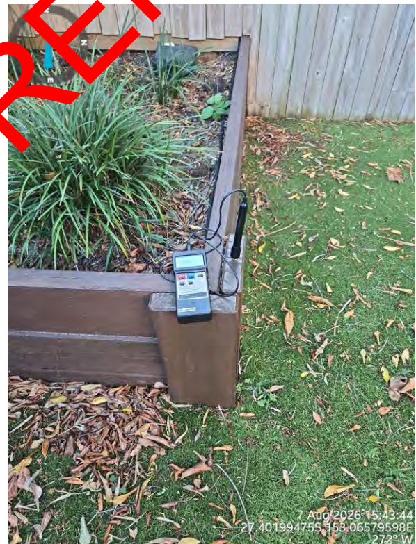
P09 - General close-up of cracked timber and open joint at the planter edge.
