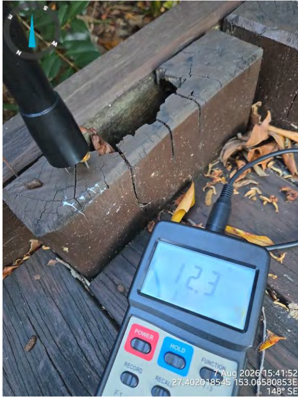
P03 - Moisture reading of 12.3% adjacent to deteriorated timber.
