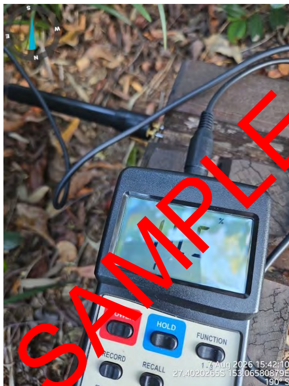
P04 - Moisture testing adjacent to a cracked exposed timber junction.
